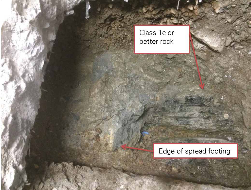
Photo No. 3 – Test Pit TP-1: View of the edge of the footing, embedded with bedrock (facing west)
